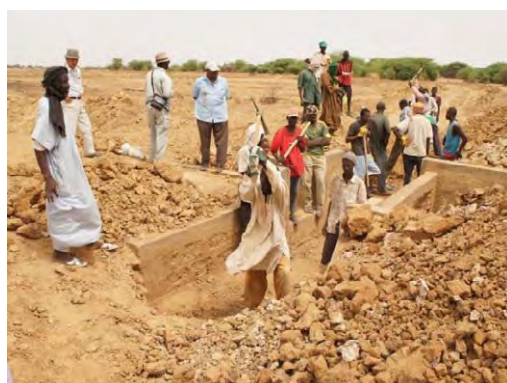
Repairing work of existing canal done by farmers' participation. June, 2011 (Podor, Korkadie area)
