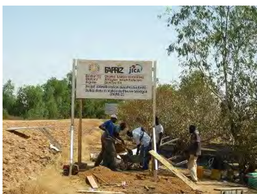
Installation work of the sign board which indicates the Project area of the repairing work for irrigation facilities by PAPRIZ. November, 2011 (Project area in Podor)
