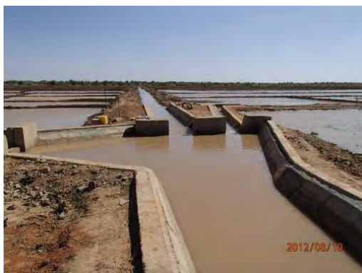
Construction work of distribution box completed by farmers' participation. March, 2012 (Podor, Diatar2 area)
