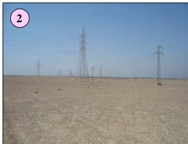
Figure A2. 5 (Al-Anbar) 400kV & 132KV Transmission Line
