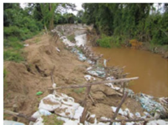
Figure 3.5.2 Destroyed river bank protection work
