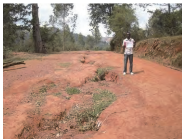
Scour observed on PR212
