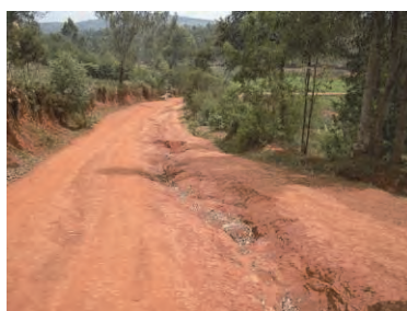
Severe scour which vehicles are possibly stuck on the road
