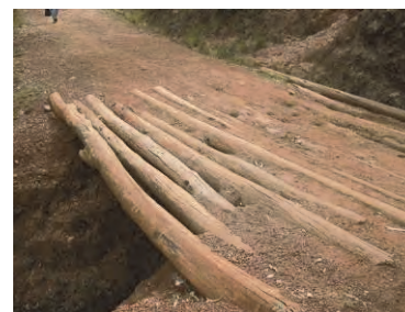
Primitive bridge may fall by water erosion in Buraza
