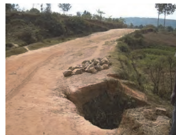
Collapse of the road beside river
