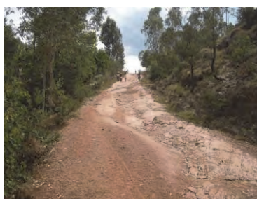
Slope severely eroded by water in Buraza
