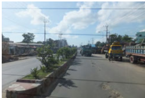
Example of Damaged Pavement (with Potholes)
