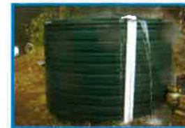
Overflowing Water Tank
