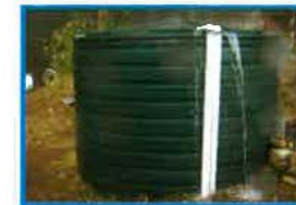
Overflowing Water Tank
