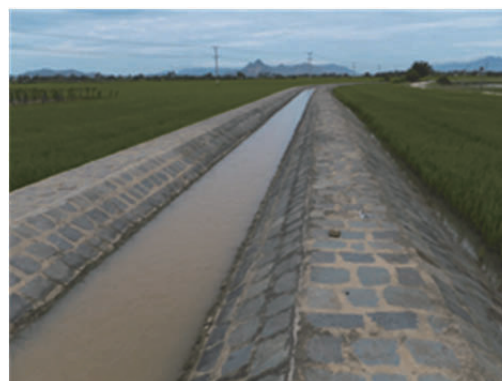
Canal constructed by Phan Rang Irrigation Project. After some rehabilitation, canals are still functioning.
