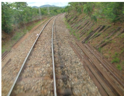
Photo 6.1: Trace of Derailment (Abandoned Rails and Bent Sleepers)
