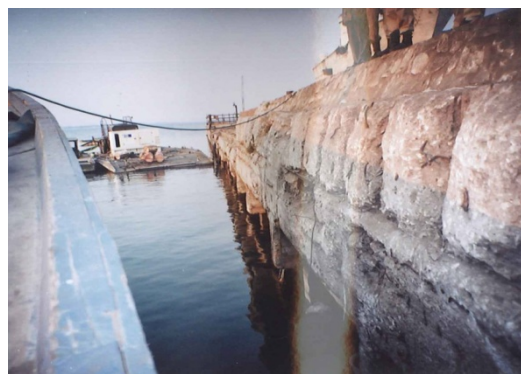
Photo 3.49: Damaged Concrete Deck and Piles (Kalemie)
