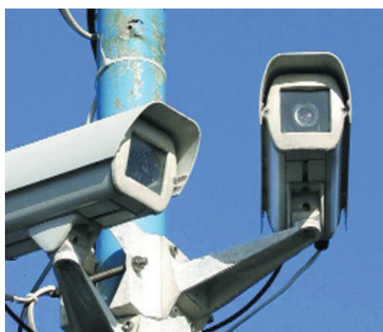
Figure 162 Example: Image of CCTV Camera
