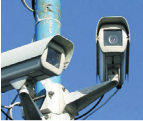
Figure 106 CCTV on Roadside
