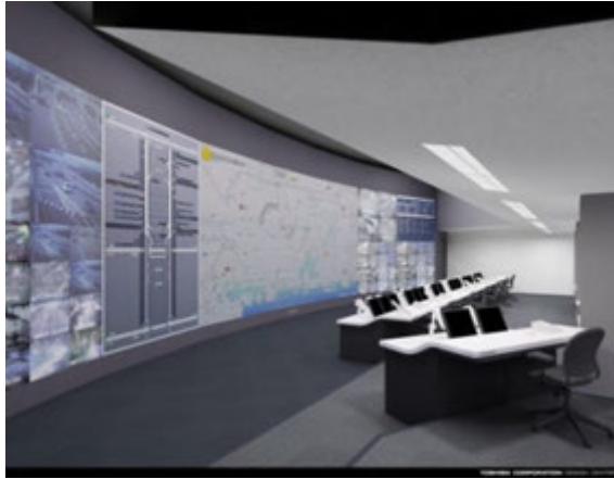
Figure 100 Traffic Control Centre
