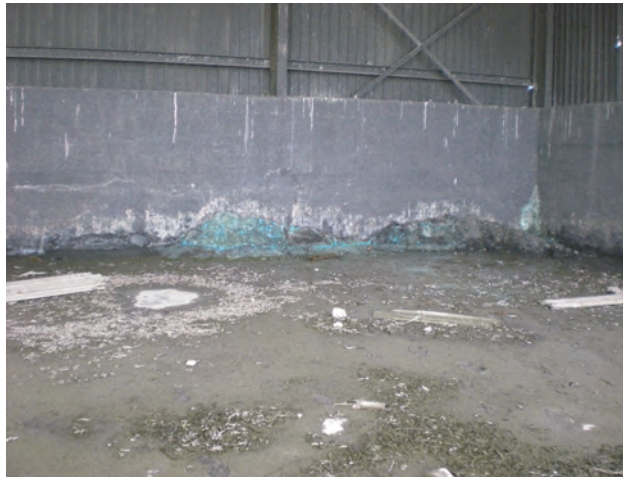
Photo 3.28 Stockpile of concentrate (Cu concentrates are remaining)
