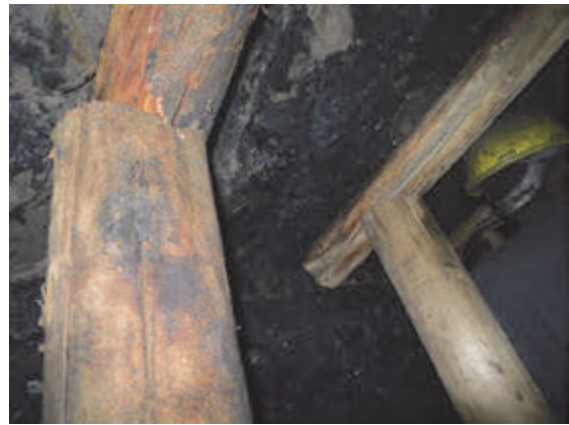
Photo 4.24 Condition of Roof in the Drift of Kaziwiziwi Coal Mine
