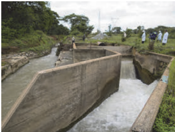
Photo 4.43 Drainage from Mine Facilities and Underground (the discharged water flows in Kafue River)
