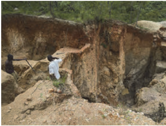
Photo 4.29 Digging by Inhabitants (they do not have PPE.)
