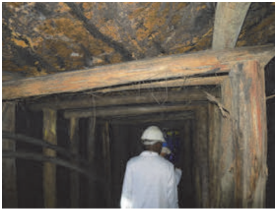
Photo 4.23 Condition of Support in the Drift of Kaziwiziwi Coal Mine
