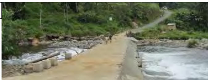
Kalasugan causeway (No Debris Flow Deposits)
