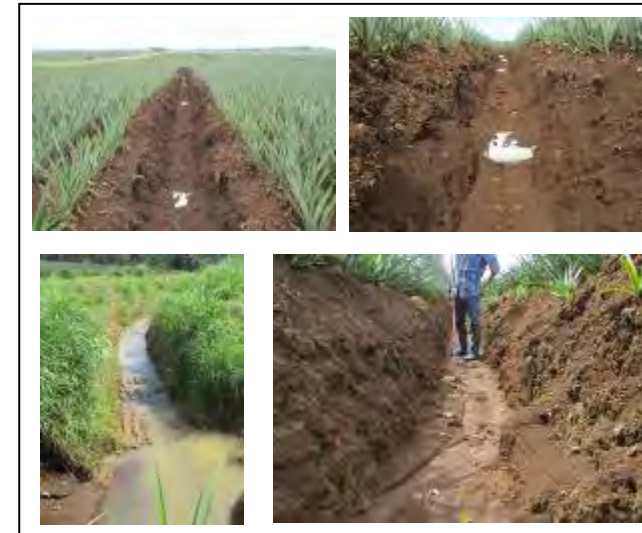
Photo 4.6.4 Channel entrenched in the Field (width : about 40cm) Upper: The Sandbags are put in the Channel for the sake of Erosion Prevention Lower (right): Trace of Outflow Lower (left): Water contains Fine Materials
