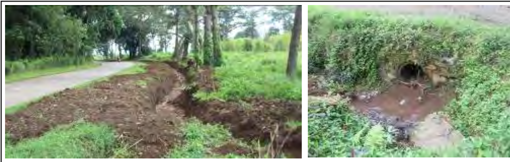
Photo 4.6.2 Unlined Side Ditch along the Road Outflow of the fine materials are observed in the Ditch
