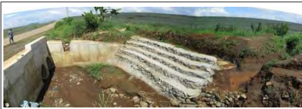
Photo 4.6.3 Retaining Wall and Drainage Culvert Deposit of Fine Materials is observed
