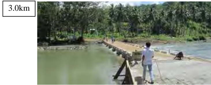
Tumalaong Causeway (No Debris Flow Deposit)
