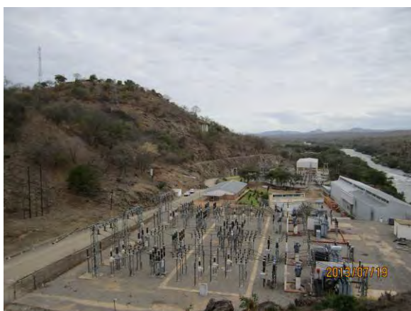
Photo-7: Existing Tedzani I, II Substation
