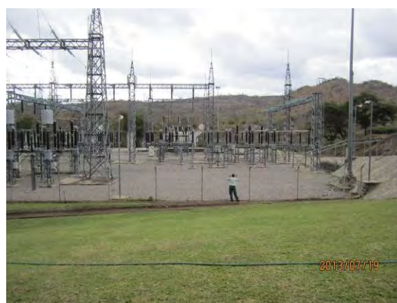
Photo-8: Existing Tedzani III Substation
