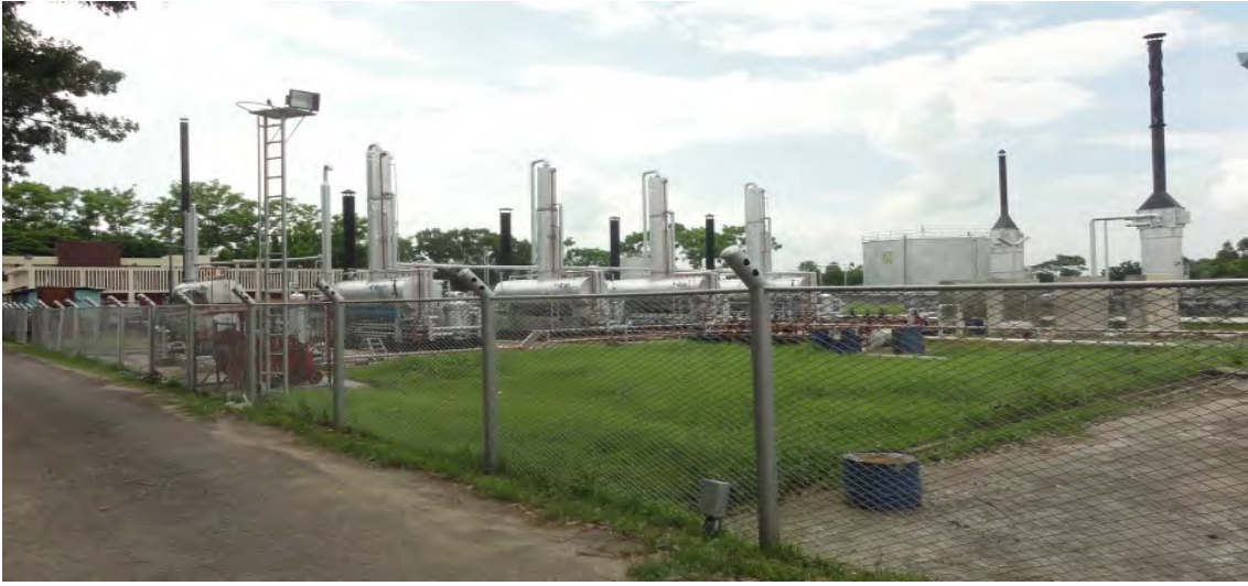
1) Overview of Titas Gas Field (Location A)
