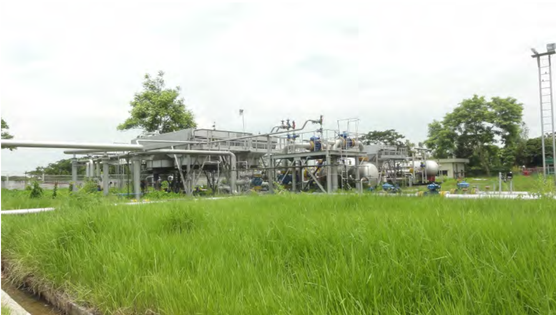
2) Overview of existing gas processing facility
