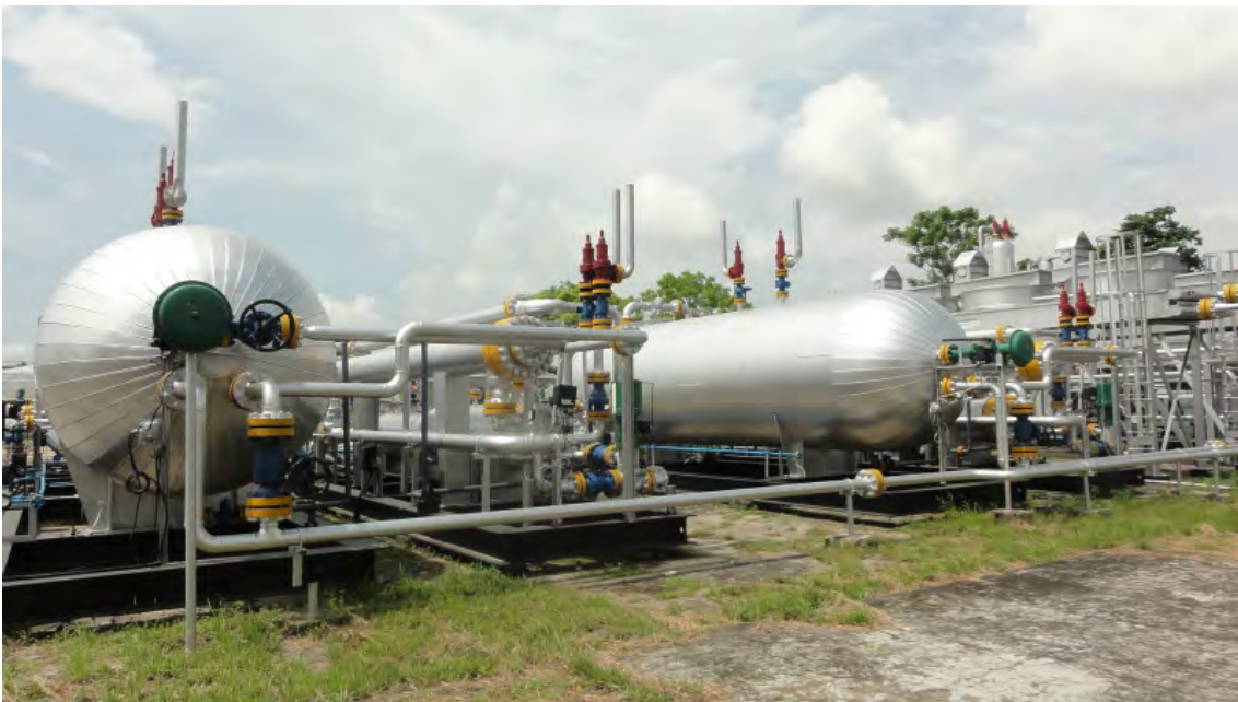
2) Overview of existing gas processing facility
