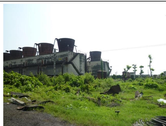
Site Survey in Existing Plant Area (Obsolete Cooling Towers of Units No.4/5)
