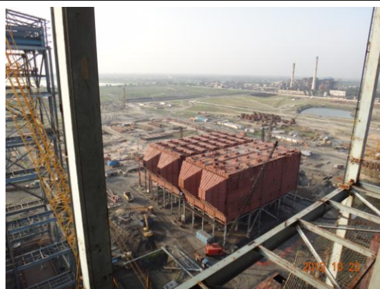
Construction of ESP of Unit No.9 (from top of Unit No.8 Boiler)
