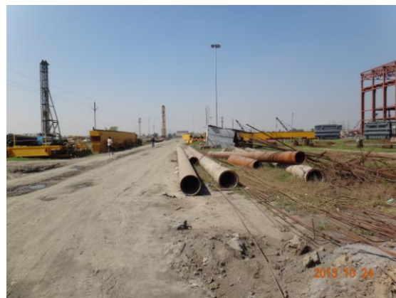
Planned Site of Unit No.10 (Used as Laydown Area of Units No.8/9 Construction)
