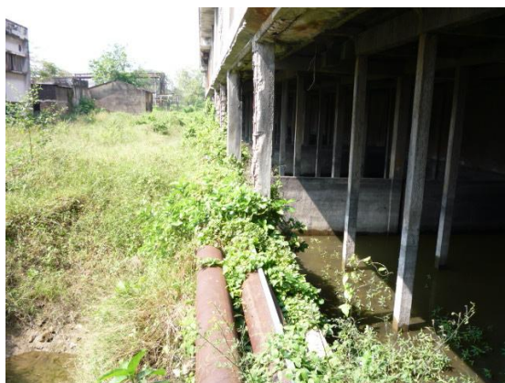
Site Survey in Existing Plant Area (Reuse: Cooling Tower of Units No.1-3)
