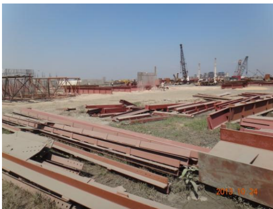
Planned Site of Unit No.10 (Used as Laydown Area of Units No.8/9 Construction)
