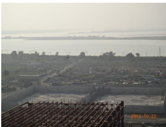
Construction of Raw Water Reservoir of Units No.8/9 (from top of Unit No.8 Boiler)
