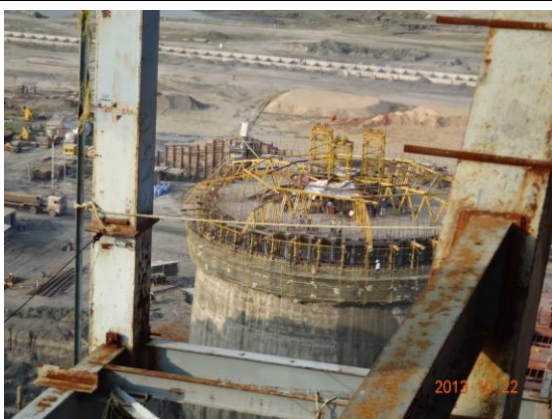
Construction of Chimney of Units No.8/9 (from top of Unit No.8 Boiler)
