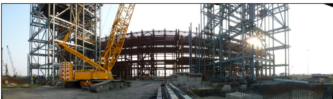
Figure 3.1-8 Construction of Units No.8/9 (Left: Unit No.8 Boiler, Right: Unit No.9 Boiler, and Center: Turbine Building)
