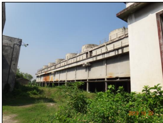
Units No.1-3 Cooling Tower
