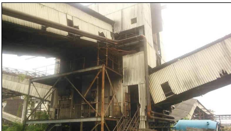
Figure 4.2-3 Current Situation of Coal Handling Equipment
