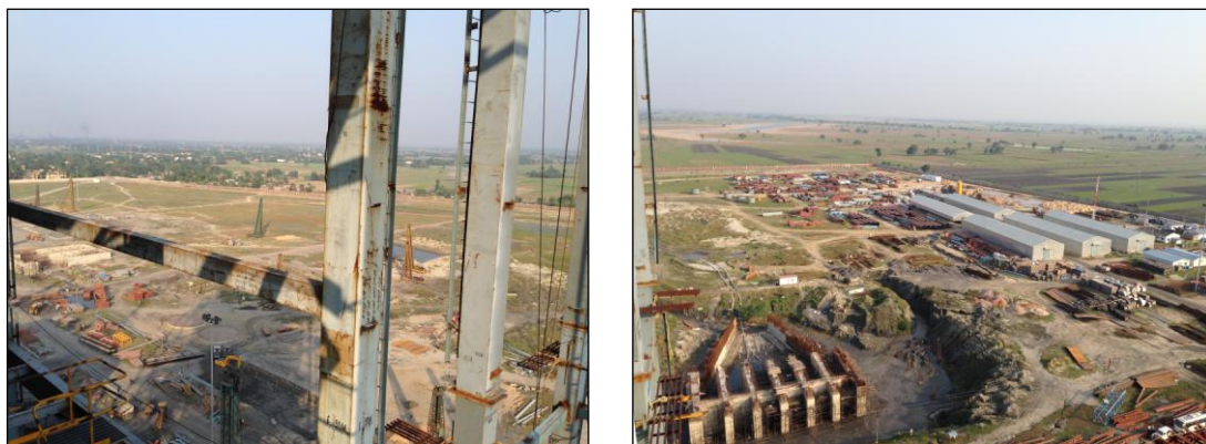
Figure 4.11-2 Northeast Side of the Barauni TPS (in the back of the Photo), Southeastern Side (in the back of the Photo)
