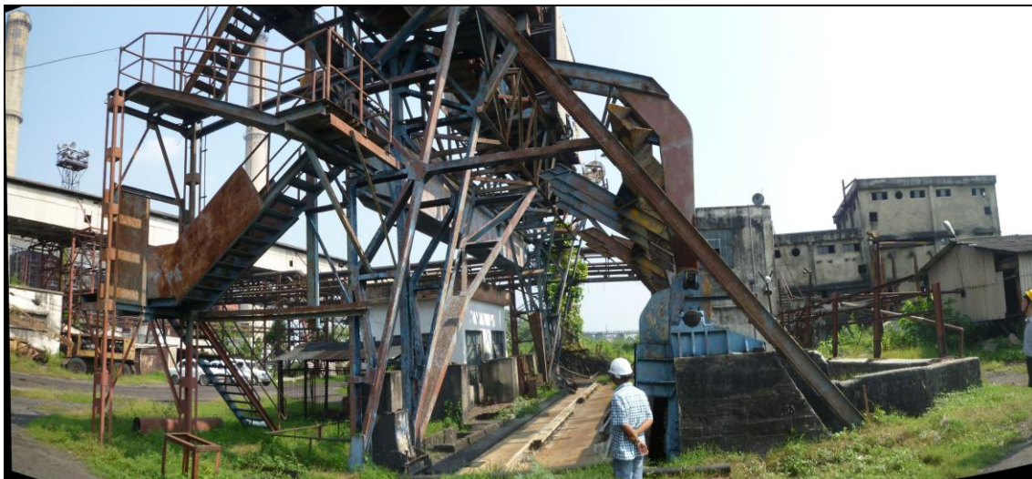
Figure 3.1-5 Wagon Tippler (Coal Unloading Equipment)
