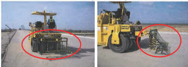
Device installation for protection of catching
