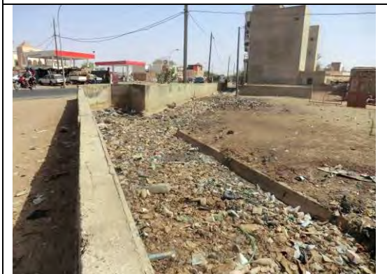
Illegal Dumping of Solid Waste and Sediment in Drain (2)
