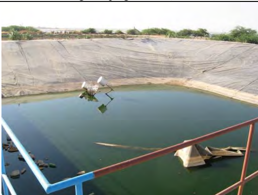
Sewage Treatment Plant (Aerated Lagoon)
