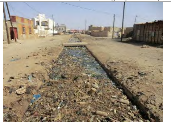
Illegal Dumping of Solid Waste and Sediment in Drain (1)
