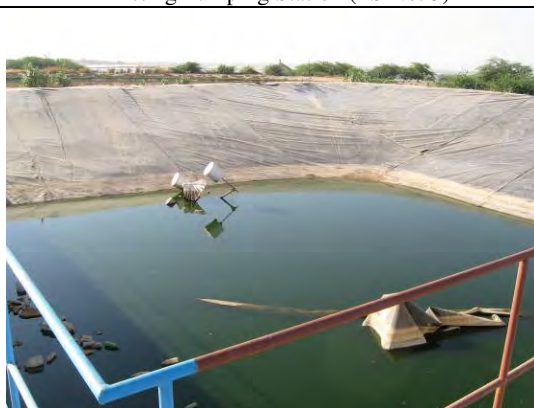
Sewage Treatment Plant (Aerated Lagoon)
