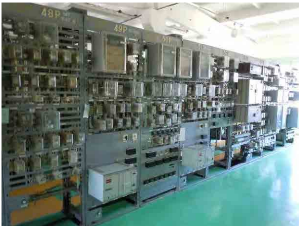
Relay Panels and Mechanical Relays
