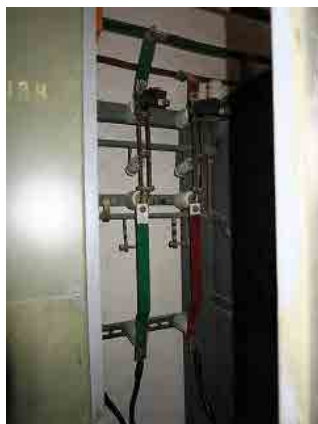
Figure 5-14 Disconnector (unavailable as a load breaker)
