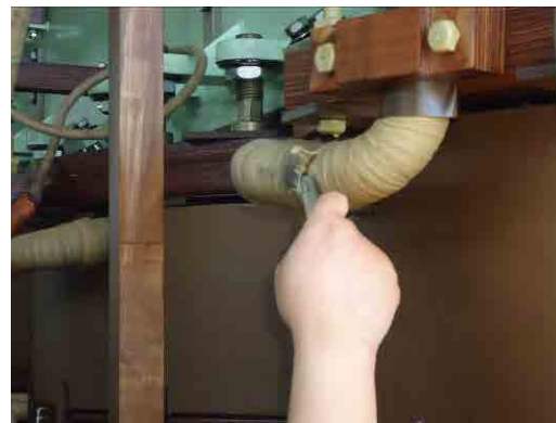
Faulty Portion of Transformer
