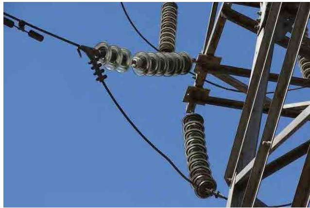
Figure 4-4 110 kV Insulators of the Incoming Tower for Baruun Substation
