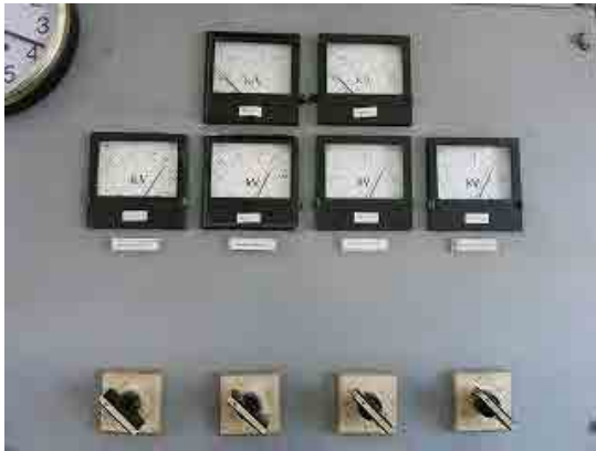
Figure 5-8 A panel in S/S (Measure of voltage to ground and interphase voltage on each feeder)
