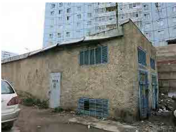
Figure 5-10 Exterior of Switching Sta. (PII13)
