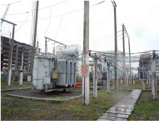
Aged Substation (Transformer and Busbar)
