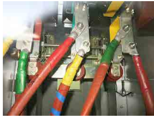
Figure 5-9 Cable Termination of Feeders (Made in Russia)
