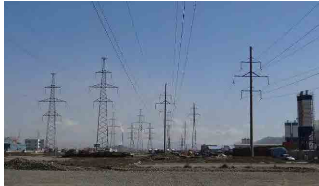
Figure 4-2 Overhead Transmission Lines near the 4 th TPP
