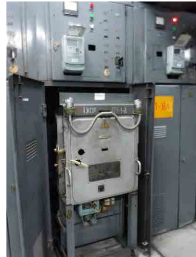
Cubicle of Russian Manufacturer
