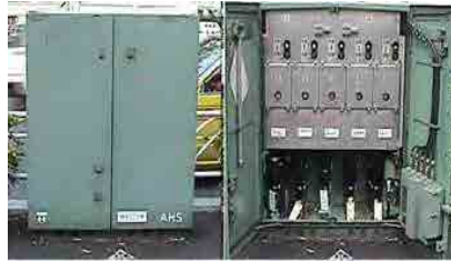
Figure 8-11 Image of Pad Mount Type Automatic Switch
