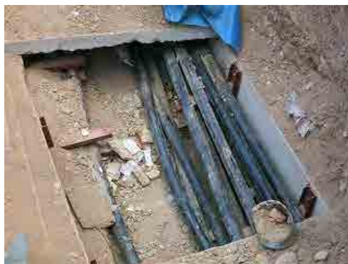
Figure 5-3 Underground Distribution System
