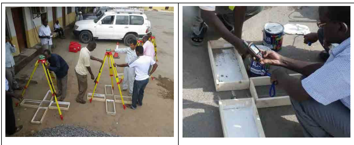
Figure 44 Technology Transfer for Reconnaissance, Selection and Installation of Control Points (Left: GNSS Antenna Installation; Right: Handy GPS Operation)
