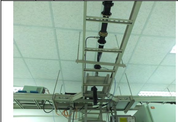
Radar equipment room: 6F (Wave-guide Configuration)
