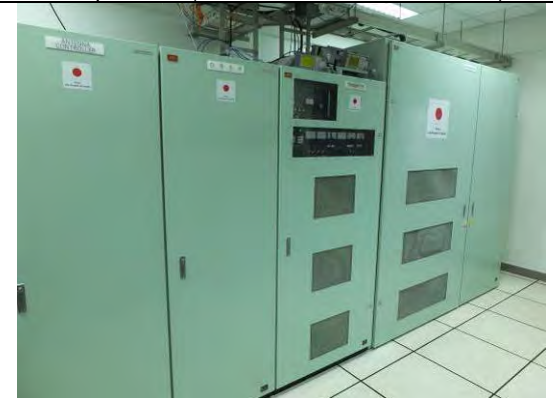
Radar equipment room: 6F (Transmitter, Digital Receiver and Signal Processor and Antenna Controller)
