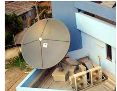
Antenna of Existing Meteorological Satellite Data Receiving System
