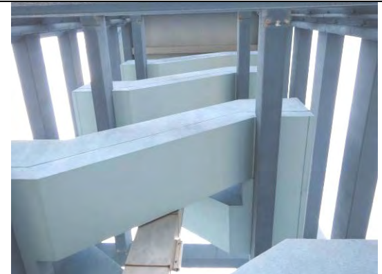
External stair soffits painted under JICA follow-up cooperation (the end of 2011-March 2012)
