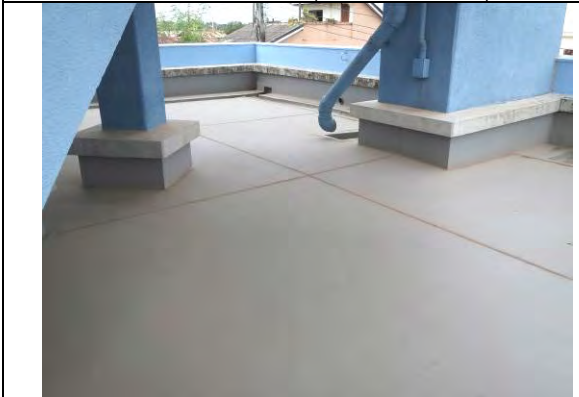
Water proof seat on 2F roof constructed under JICA follow-up cooperation (the end of 2011-March 2012)
