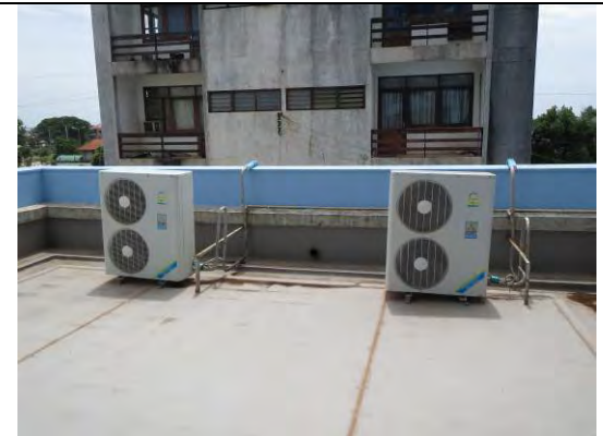
Exterior unit of air conditioners (2) newly installed at the weather forecasting room by the Ministry of Natural Resources and Environment
