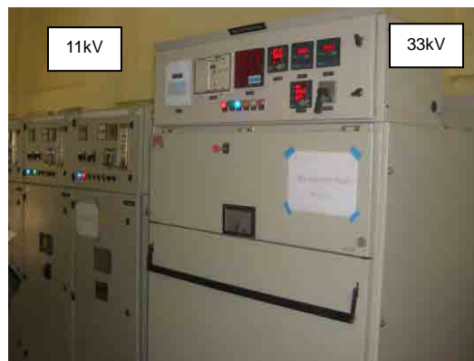
Figure 2-19: 33kV and 11kV Switchgear
