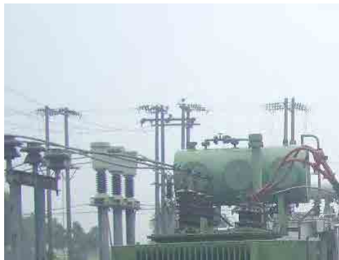
Figure 2-10: Khayaebin substation and 33kV transmission lines
