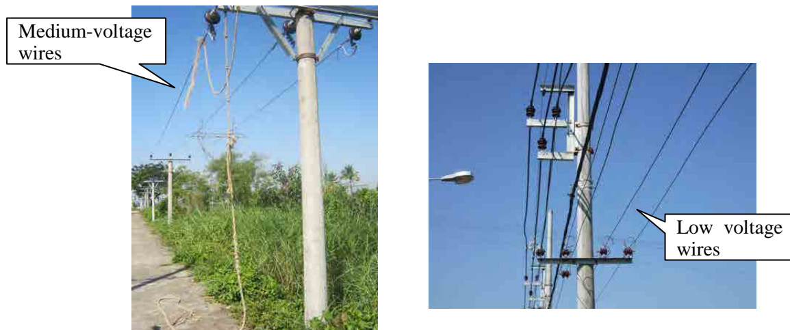
Figure 5-10: Practical training facilities (Distribution overhead lines and poles)
