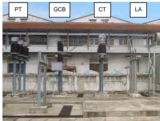
Figure 2-18: 66kV PT, GCB, CT, LA
