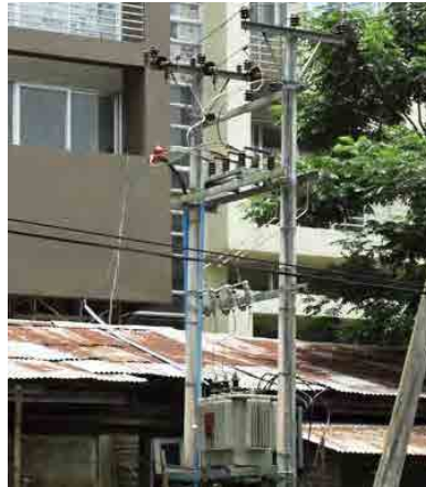
Figure 2-20: Transformer with a set of drop out fuses, disconnection switches and arrestors mounted on two poles
