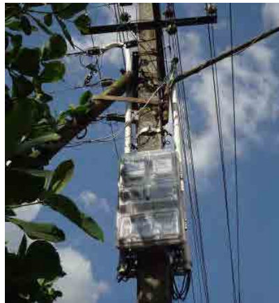
Figure 2-22: Offsite meter reading system on a pole
