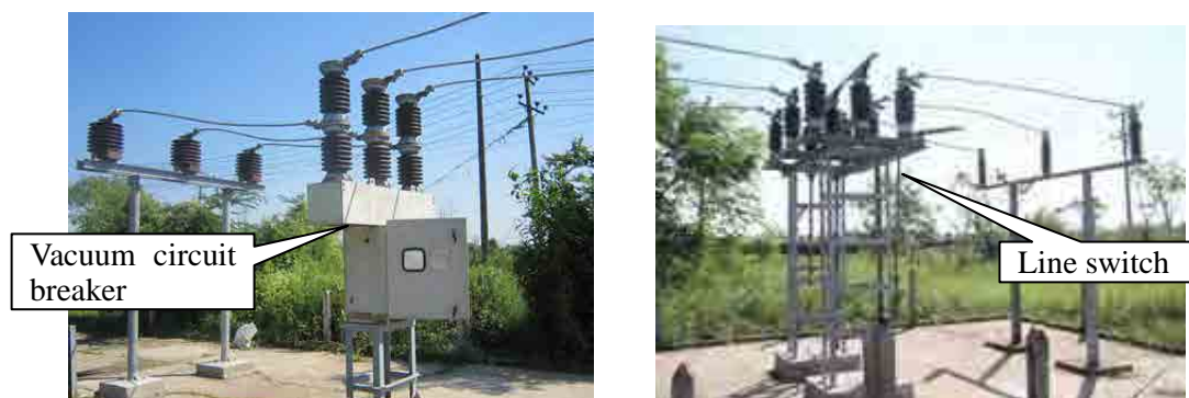
Figure 5-11: Practical training facilities (Substation facilities)
