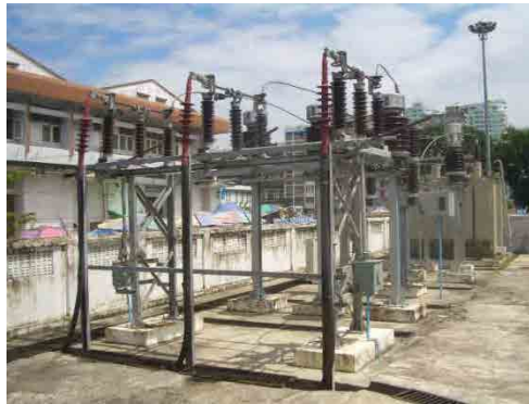
Figure 2-9: Cable head for 66kV transmission line service entrances at Mawtin substation
