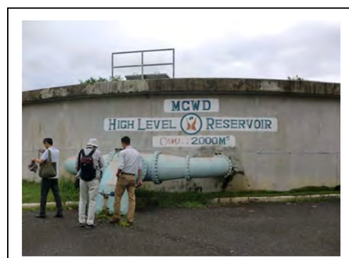
写真-3 Liloan (High Level)配水池
