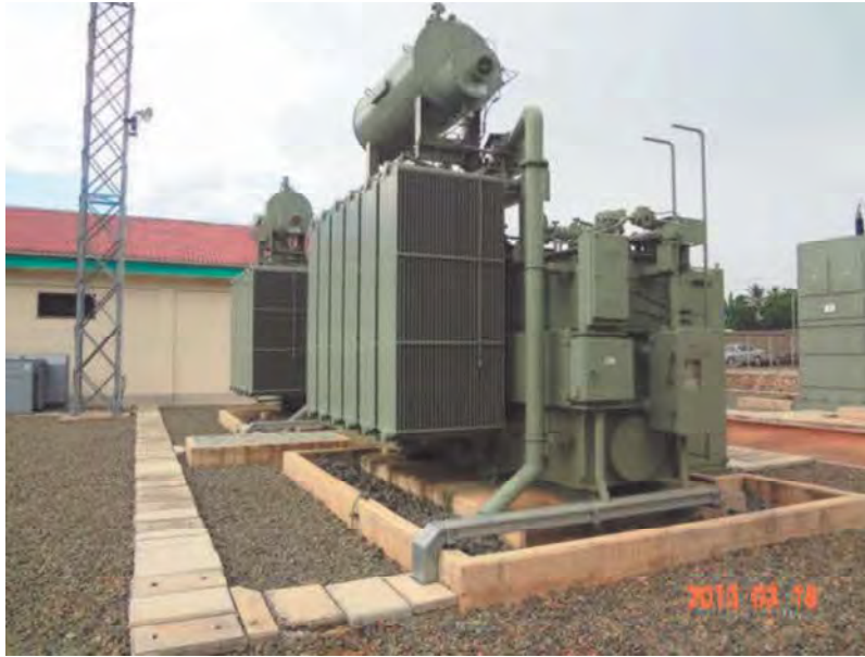
Figure 0 15MVA transformer for 33/11kVsubstation
