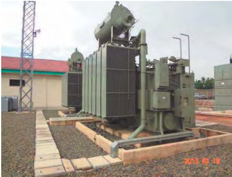
Figure 0 15MVA transformer for 33/11kV substation
