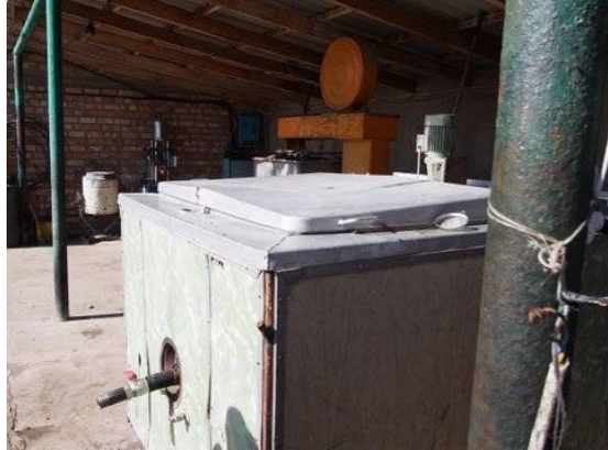
Picture2-19 Bulk Cooler
