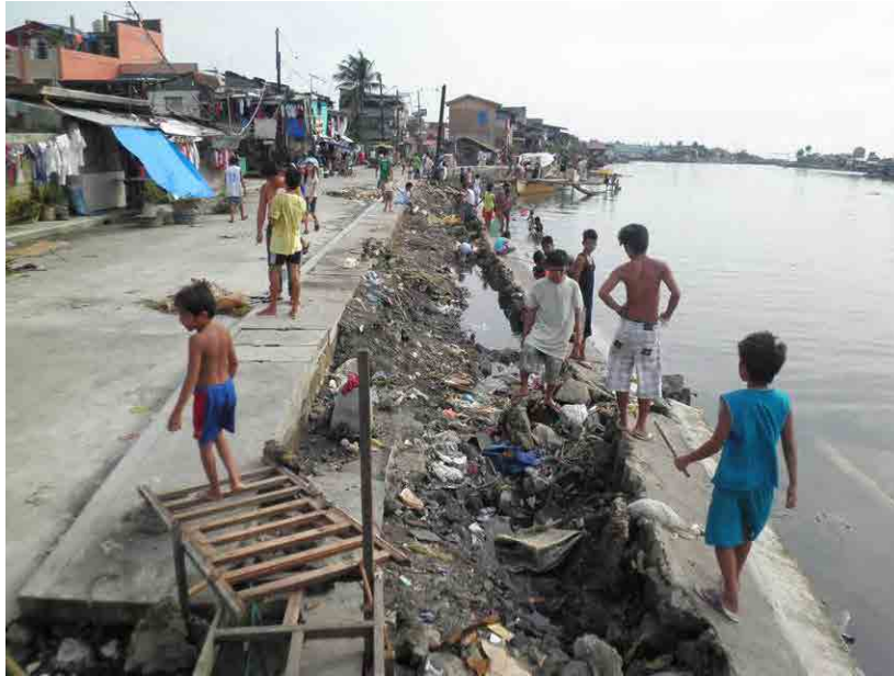
Figure 5.10.4 Photo of Collapsed River Wall at Left Bank of Marala River
