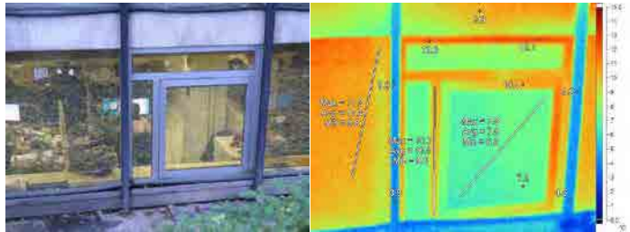
For Building A and B, Heat loss through window and sash is high, Not closing blinds
