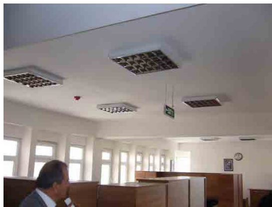
Figure 7-15 Reflector Lighting with Utilization of Sun Light
