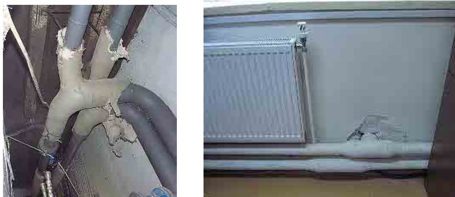
Figure 2.3.2-12 Non-insulated Pipes in Piping Shaft and Office Area in DSI Buildings
