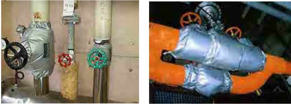
Figure 2.3.2-16 Insulation Jacket for Valves
