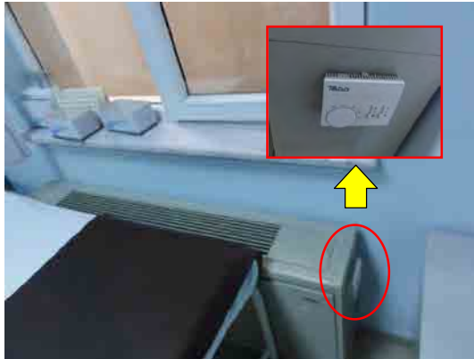
All FCU have a thermal control unit
