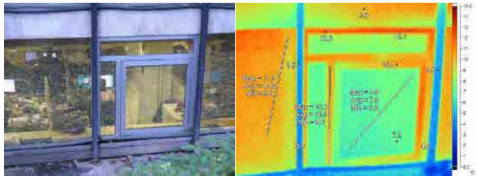
For Building A and B, Heat loss through window and sash is high, Not closing blinds
