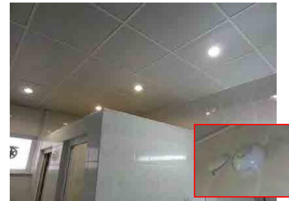
Motion sensor is installed at WC, but lightings are kept turned on
