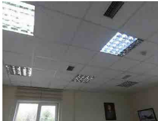
Some lighting circuits are separated → Easy to select the lighting area
