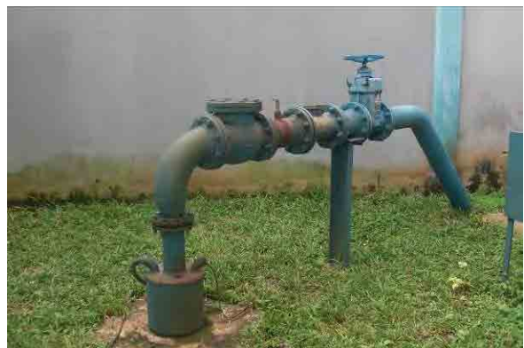
July 2013, Field Survey (Lagos Water Service with Well)
