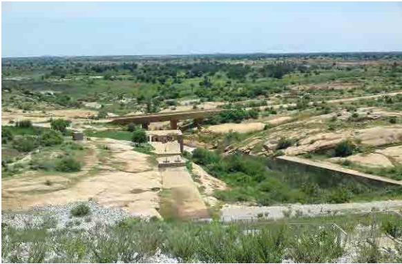
September 2011, Field Survey (Challawa Dam)
