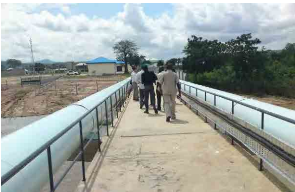
September 2011, Field Survey (WTP in Lokoja)
