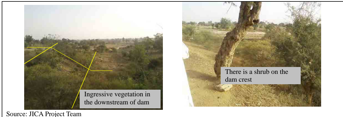
Photo-1 Intrusion Status of Vegetation in Zuru Dam Body
