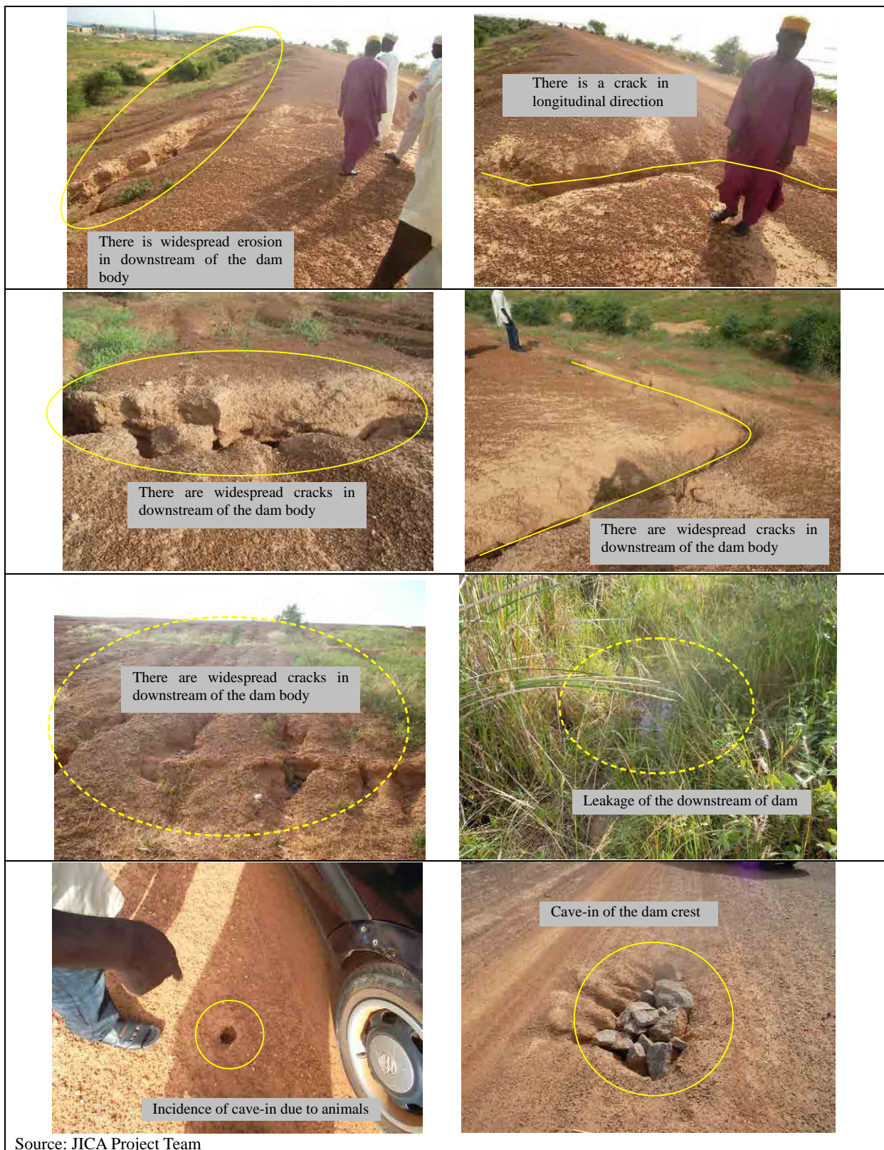
Photo-3 Erosion and Leakage Status in Stream of Watari Dam Body
