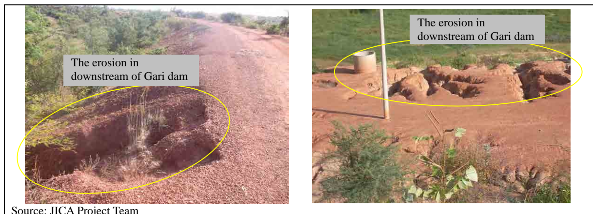
Photo-2 Erosion Status in Gari Dam Body
