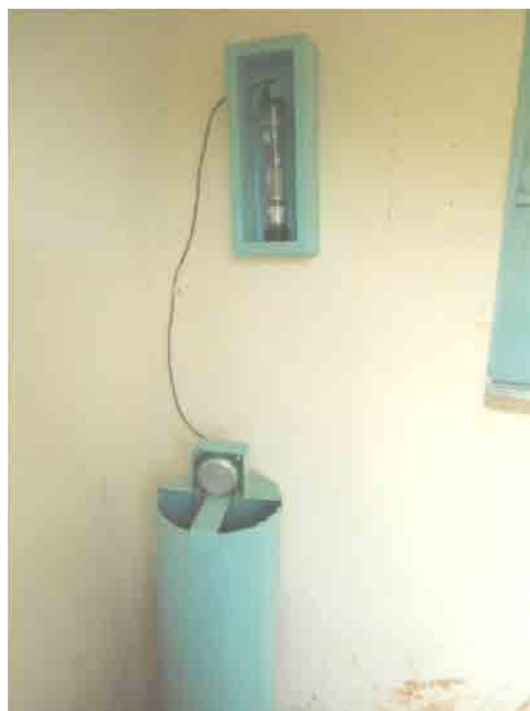
Figure 11: Ott Thalimedes Data logger installed in a data logger house
