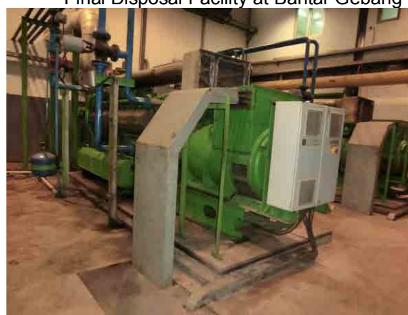
Methane Gas Recovery and Power Generation Facility at Bantar Gebang
