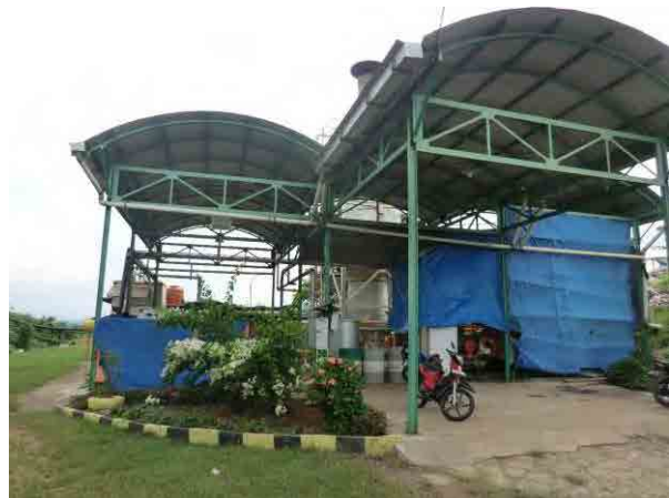
Methane Gas Recovery and Power
