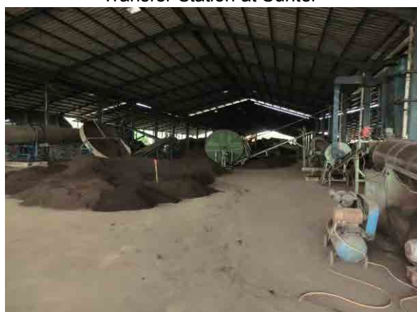
Compost Facility at Bantar Gebang
