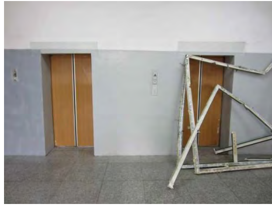
Photograph: An elevator made unusable due to leaning of the framework
