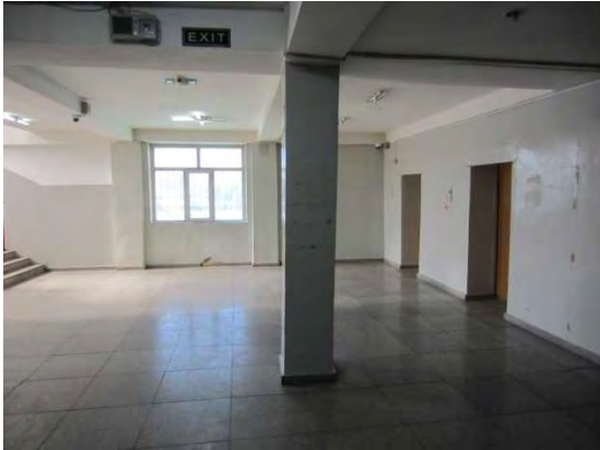
Photograph: A leaning pillar in the elevator hall
