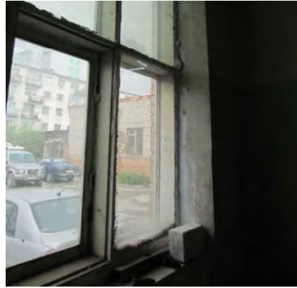
Photograph: A window which has not been renovated
