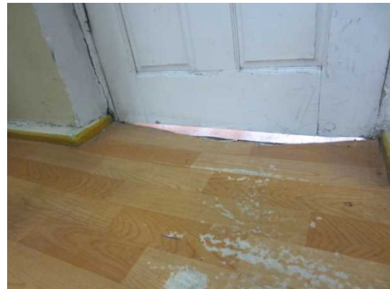
Photograph: A large gap under a door created by warping of the floor
