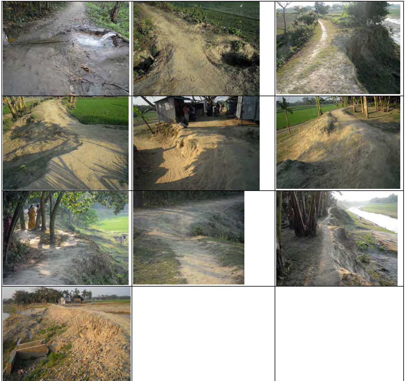
Artificial cutting and erosion due to heavy rainfall and overtop
