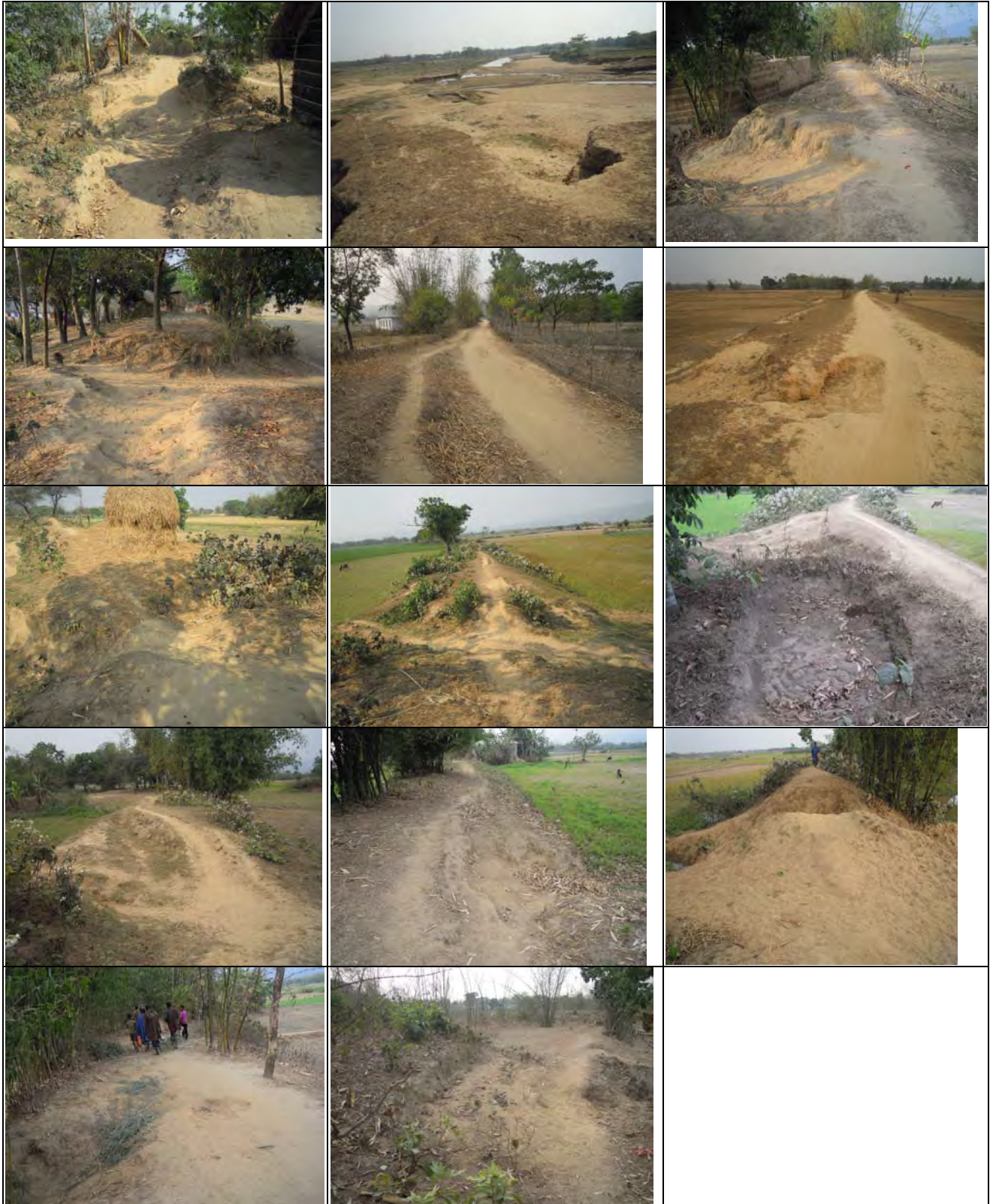
Artificial cutting and erosion due to heavy rainfall, overtop
