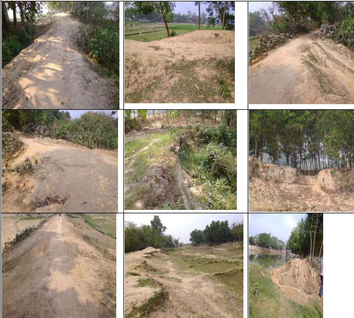
Erosion due to wave action and heavy rainfall
