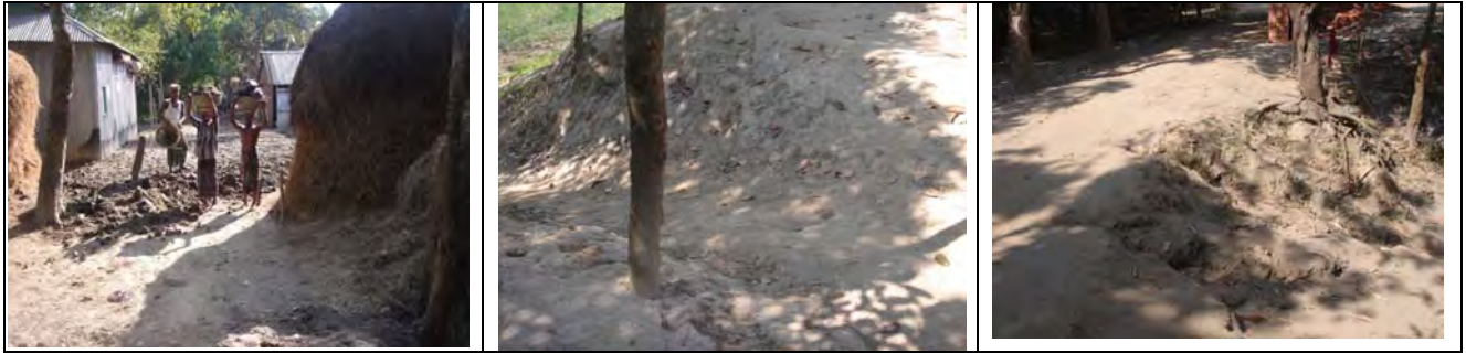
Erosion due to heavy rainfall
