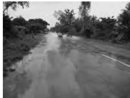
Poor Drainage (KP 57)
