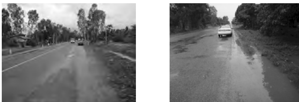
Figure 4.2-2 Road Surface Lower than Adjacent Land and Inundated Road Surface
