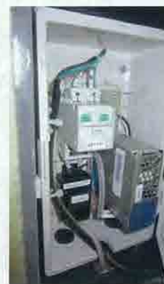
Fig 7 : Inverter in good condition
