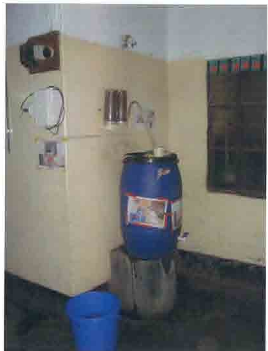
Fig6: UV water tank
