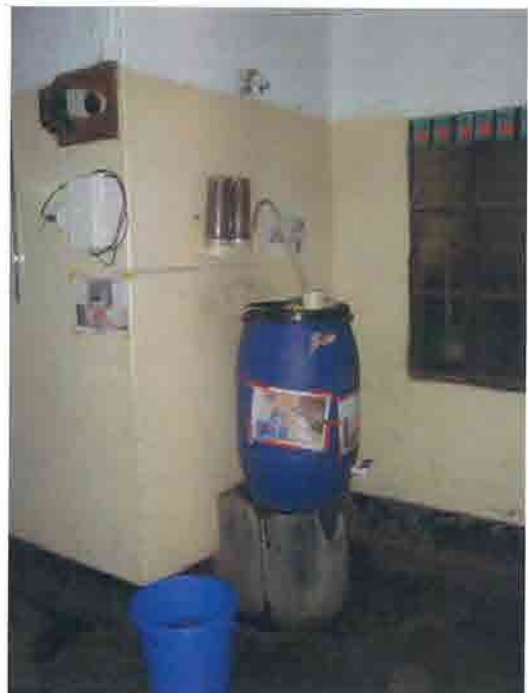
Fig6: UV water tank
