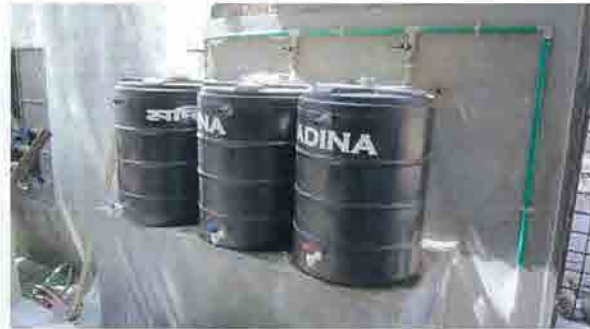
Fig 4: UV water tank
