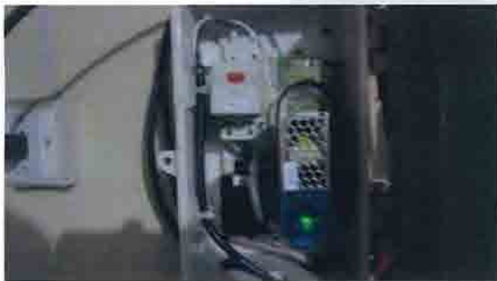
Fig : Inverter ok
