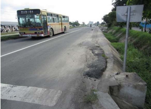
Flow rutting with large scale on outside lane of carriage way
