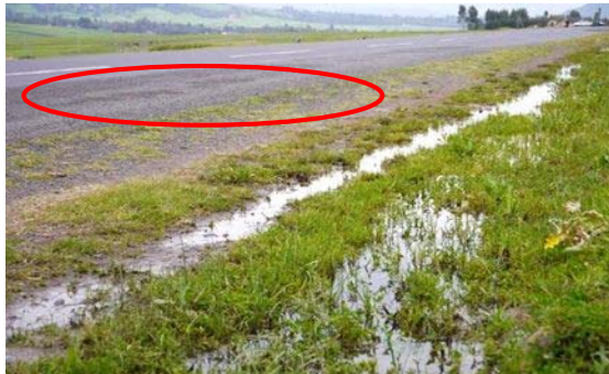
Photograph 4-1. Groundwater flowing down from the mountain side becomes the pavement failure of the mountain side carriage way. Improvement of the drainage by upsizing of the gutter or the Calvert setting is necessary.
