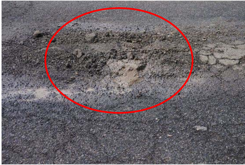
Photograph4-14. The asphalt pavement that muddy water eructs by pumping from base course.
