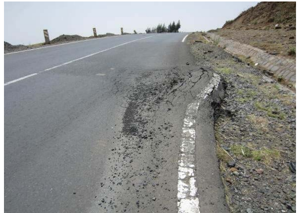
Damaged section where is identified at cut area, it may also be responded by ground water.
