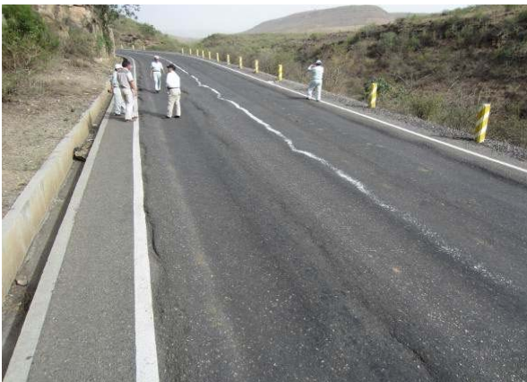
Flow rutting was identified at lowland in Abay, because of high temperature and heavy vehicle with low speed.
