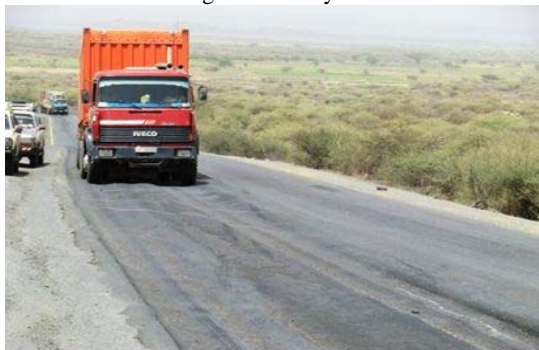
Photograph 4-3. For example rutting caused by fluidization of the surface course. Rutting is remarkable partly in the steep gradient section, because run speed becomes the super low speed.
