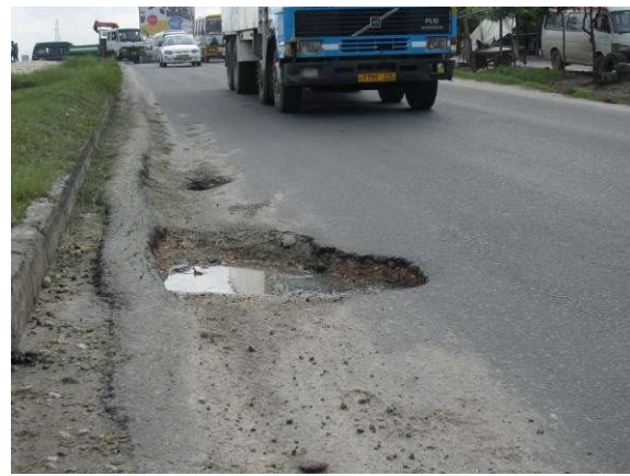
Large pot hole and flow rutting on straight section This phenomenon may be caused from thin layer with flow rutting.
