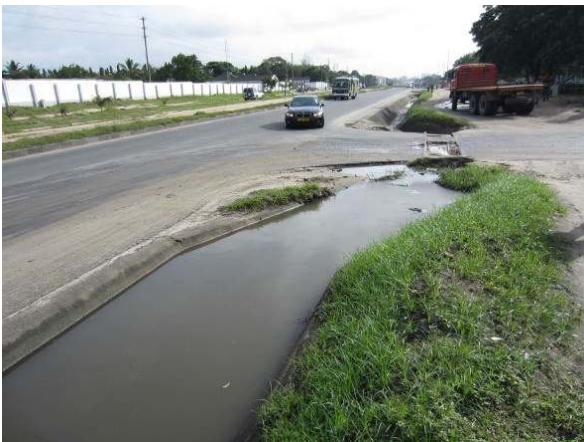
Side drainage was filled with water because of breakage of crossing pipe.
