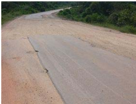
Photograph4-10. Ghana : Rural trunk road(2007) Intensive section of the surface water
