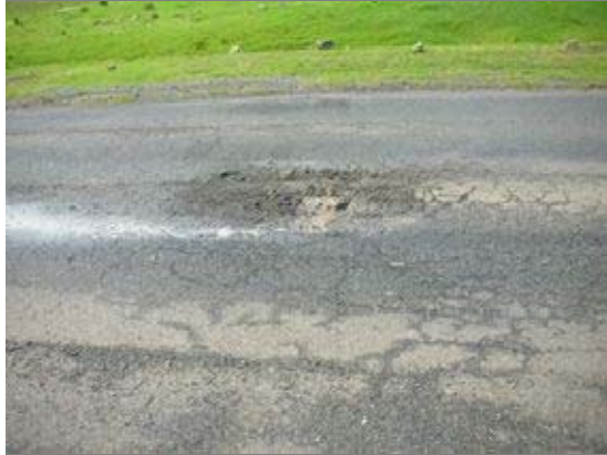
Photograph4-8. Ethiopia:Rural trunk road Pavement was failure because bearing capacity is down by influence of the water at sag point.
