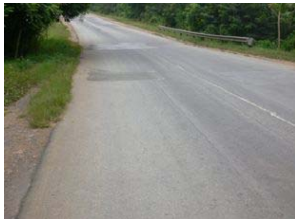
Trace of repair at sag point
