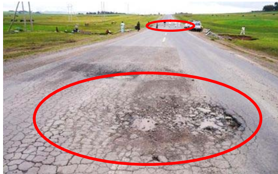
Photograph 4-2. Water in base course is mainly saturated in the sag part of the vertical section, becomes the pavement failure. Damage is seen in both sides across the bridge.
