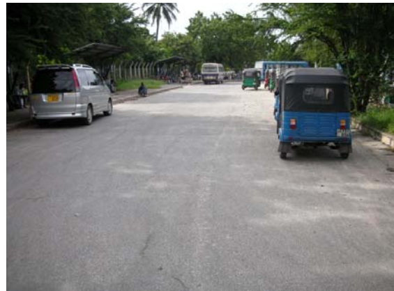
Bus Bay along Kawawa road, Semi-flexible pavement was adopted for huge number of buses.
