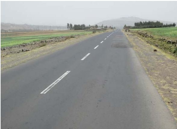
Damaged section where has large catchment area, it may be responded by ground water.
