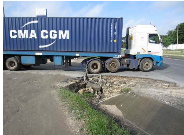
Same as left photo. Downstream side of crossing pipe was blocked with broken piece of pavement.
