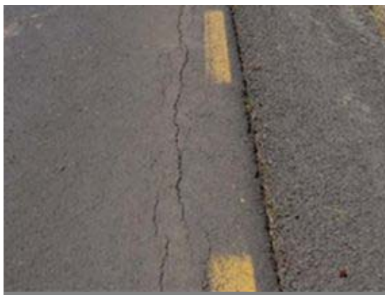
Photograph4-12. Ethiopia : Rural trunk road Typical early case of the pavement failure by black cotton soil (Vertical rutting of pavement edge)
