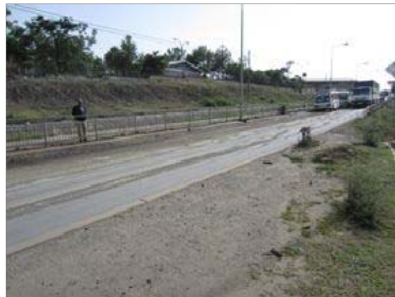
Photograph4-11. Ethiopia : Urban trunk road Under the influence of black cotton soil, Rutting occurred on the surface.
