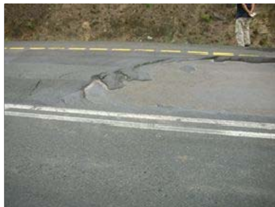
Photograph4-13. Tanzania : Rural trunk road Tack coat defects. Pavement exfoliates for heavy vehicle load
