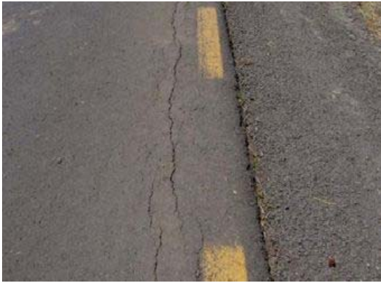
Photograph4-18. Typical early case of the pavement failure by black cotton soil (initial stage)
