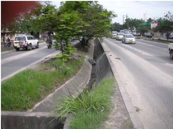
Center drainage on median strip, drainage system was carefully designed.
