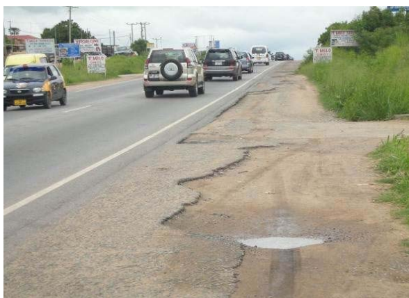
Shoulder pavement destroyed by traffic for small access road, because of thin layer (DBST)
