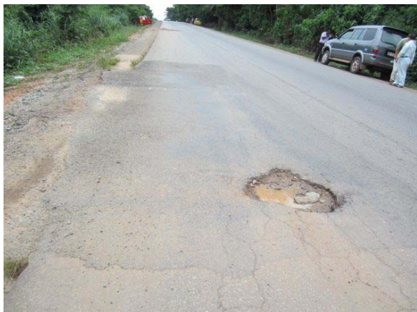
Reappeared pot hole on repaired section
