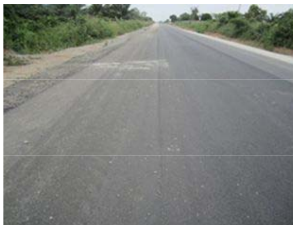
New surface As pavement under construction by Japanese ODA, As content of 5.1% is relatively high.
