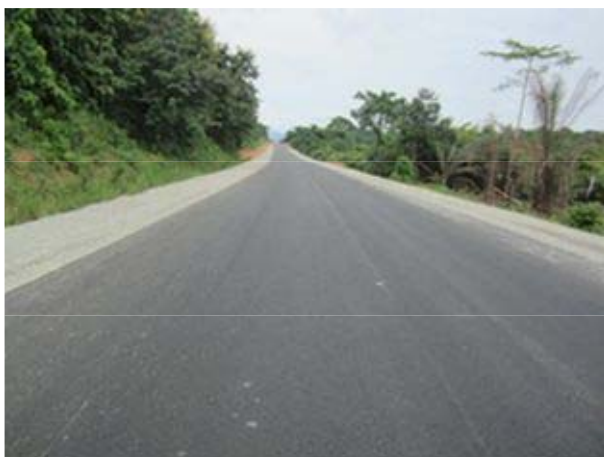
New As binder course under construction by Japanese ODA, qualities such as flatness are high.
