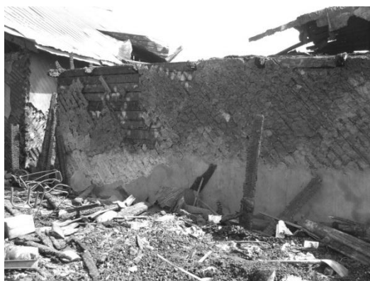
Figure 5.5.18 North side wall of burned house 1
