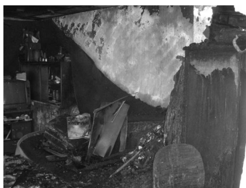
Figure 5.5.21 Inside of house was fully burned
