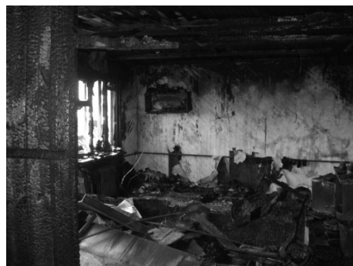
Figure 5.5.27 View of inside of house 2 (2)
