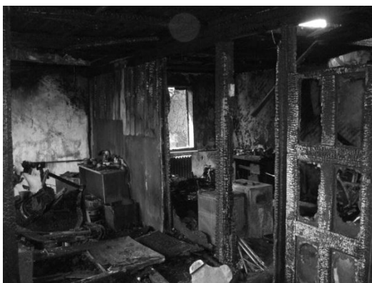
Figure 5.5.26 View of inside of house 2 (1)
