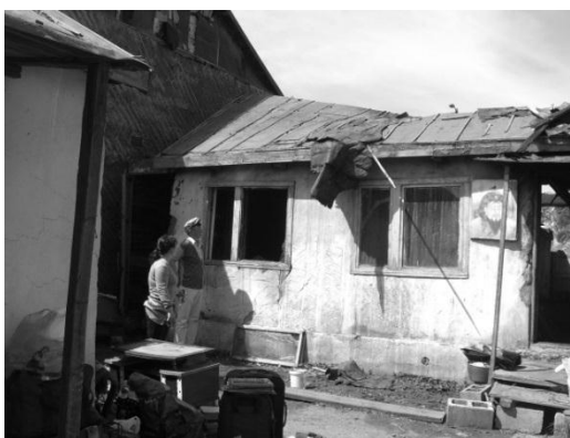
Figure 5.5.19 Southside of burned house 1
