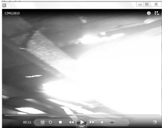
Figure 5.5.22 Ceiling and roof was burned out
