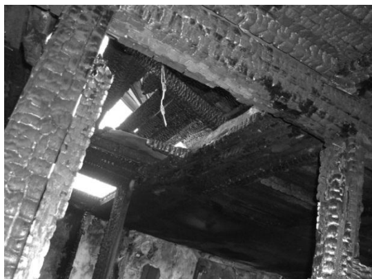
Figure 5.5.28 Look sky through burned Ceiling
