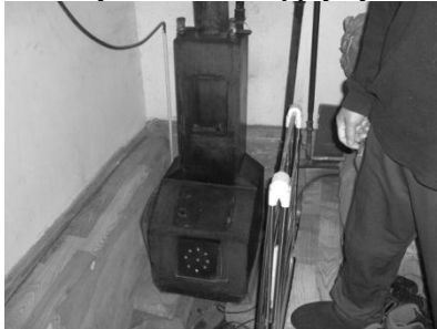
Figure 5.5.4 Hot water supply system in Ger
