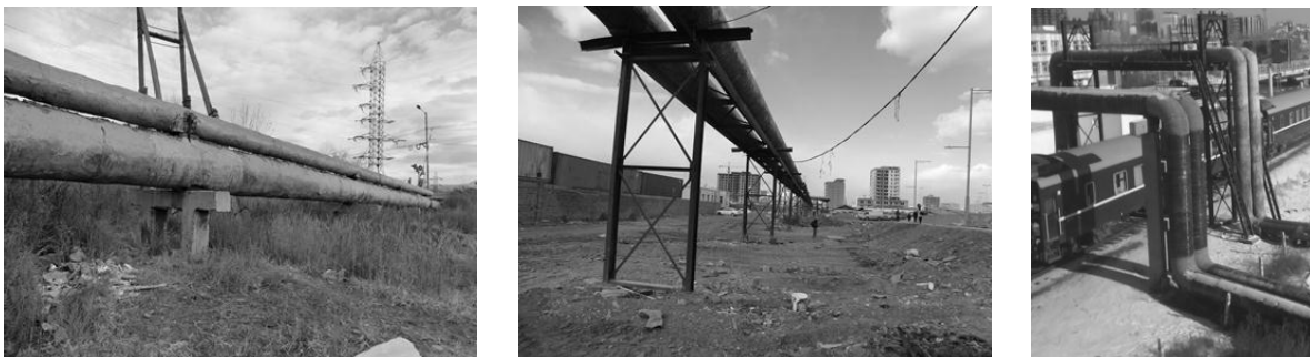
Figure 5.4.17 Over ground hot water pipeline
