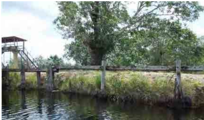
PH21-29 Rotten wooden sheet piles and the self-standing embankment slope
