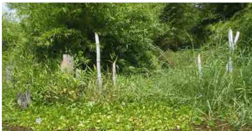
PH2-1-15 Debris of the revetment and vegetation on the slope
