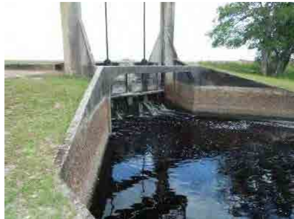
PH2-1-28 Leakage condition through the gate
