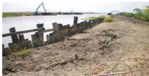
PH 2-1-4 Step, cracks and inclined revetments
