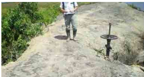
PH2-1-18 Lean and narrow embankment crest
