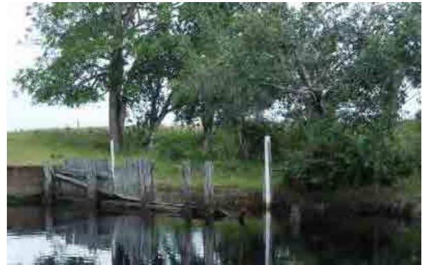
PH2-1-30 Rotten wooden sheet piles and the stable ground surface
