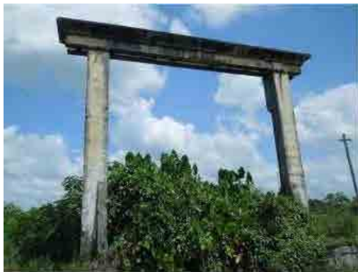
PH2-1-22' Piers for winching the Cuhnia regulation gate
