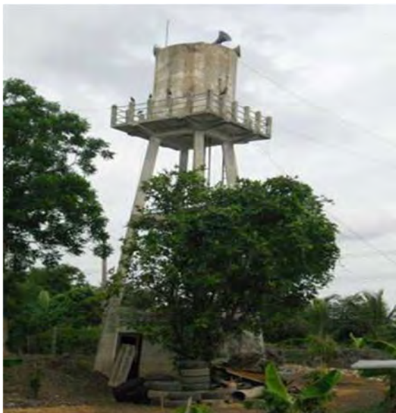
Water storage for village tap water
