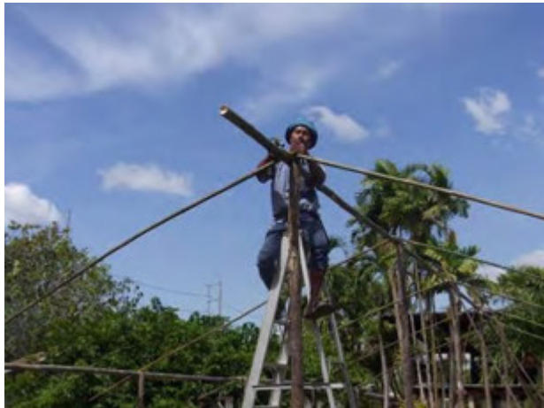
Frame structure is being assembled mainly by men. A carpenter took care of the technical part at high place. (Dec. 23, 2012)
