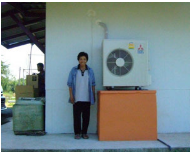
The Condensing unit outside packing house (By JICA Supporting)
