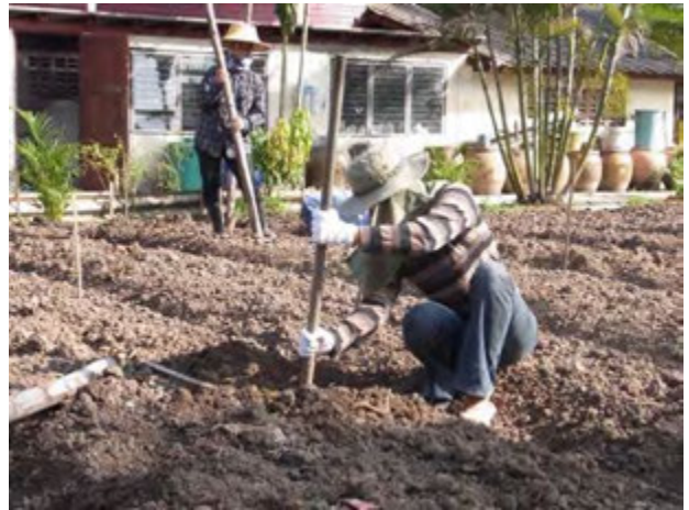
Holes for the pillars of net houses were being dug; more than 50cm in depth is recommended (Dec. 23, 2012)
