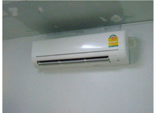
The new air conditioner in packing house room (Fan coil unit supporting by JICA)
