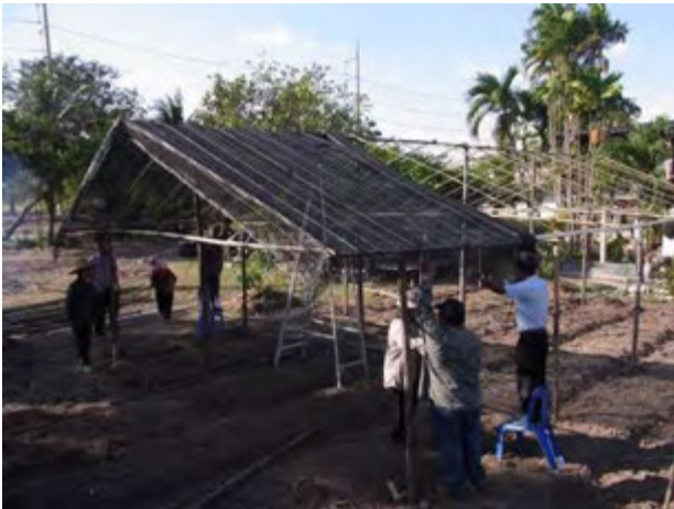
Now, putting the saran net on the roof; cooperation among people at each part is essential. (Dec. 23, 2012)
