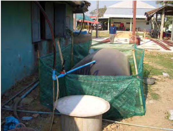
Inlet Pit and Gas Tank
