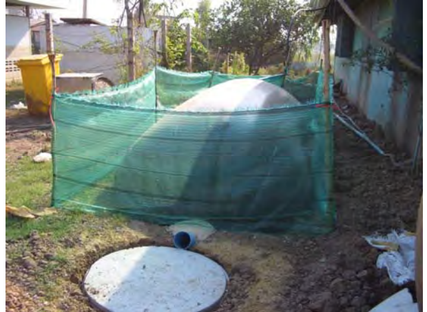
Outlet Pit and Gas Tank
