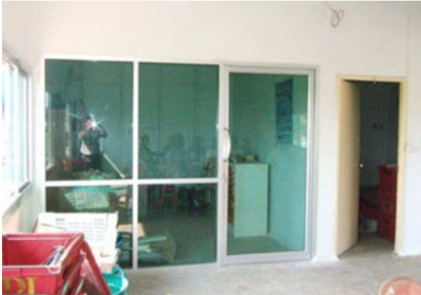
Inside packing house after Rehabilitation (By Vegetable Group Budget)
