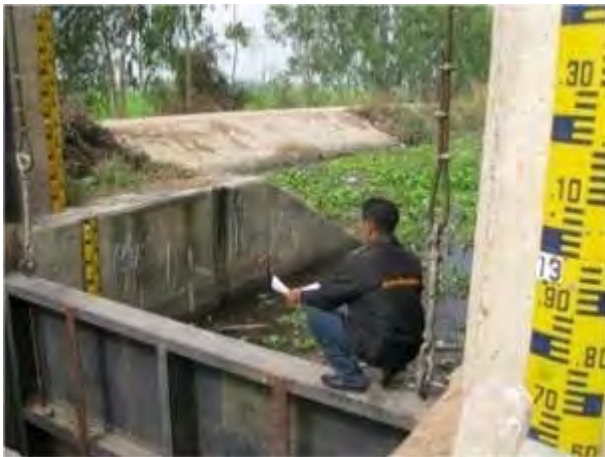
Installed staff gage
