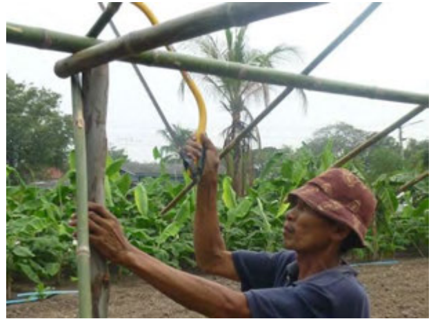
Wooden poles were employed for the pillars, while bamboos were used for roofing structure. (Jan. 30, 2013)
