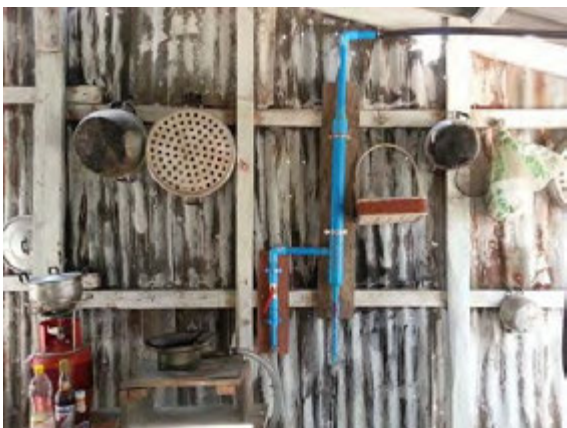
Gas Pipeline connected with stove in farmer's kitchen
