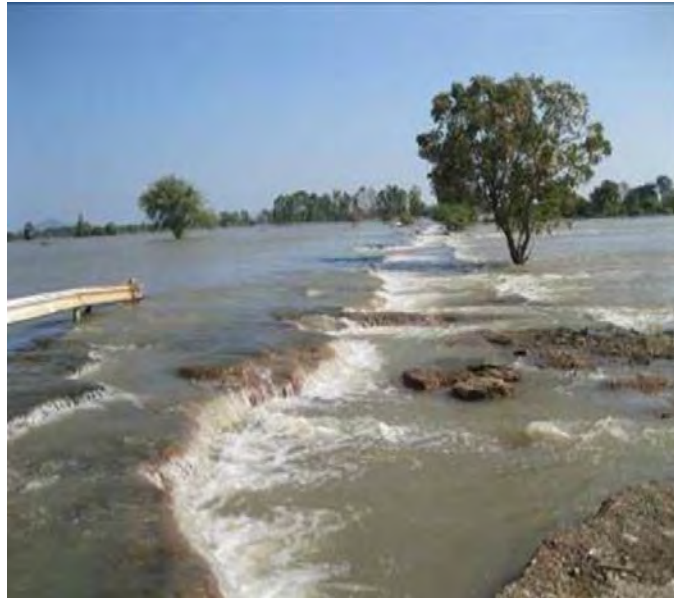
Figure 13 Road damaged by the Flood
