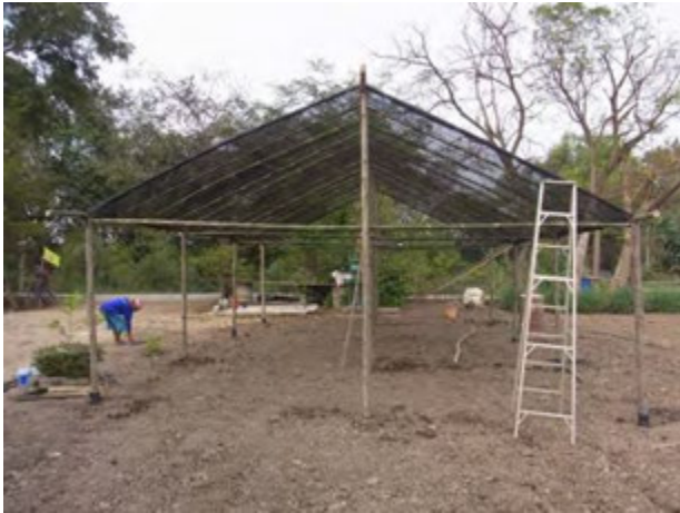
A simple net house completed; saran net roof will mitigate strong sunshine during summer time and reduce excessive rain during rainy season. (Jan. 30, 2013)
