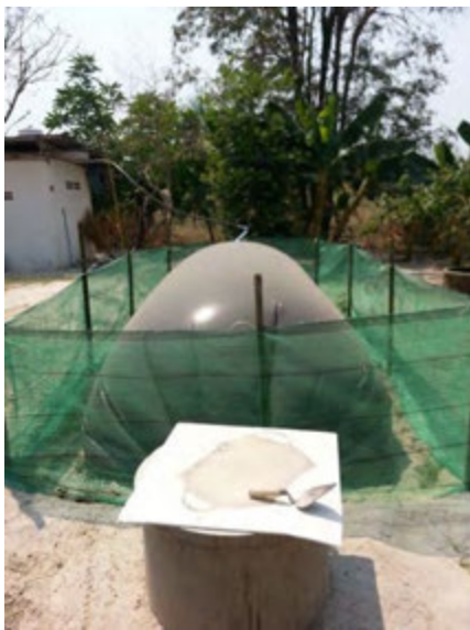
The inlet tank
