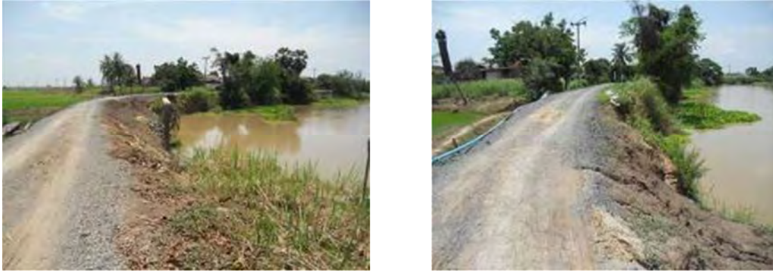
Fig: Recurrence damage of dike road along Bang Ban (Noi river)
