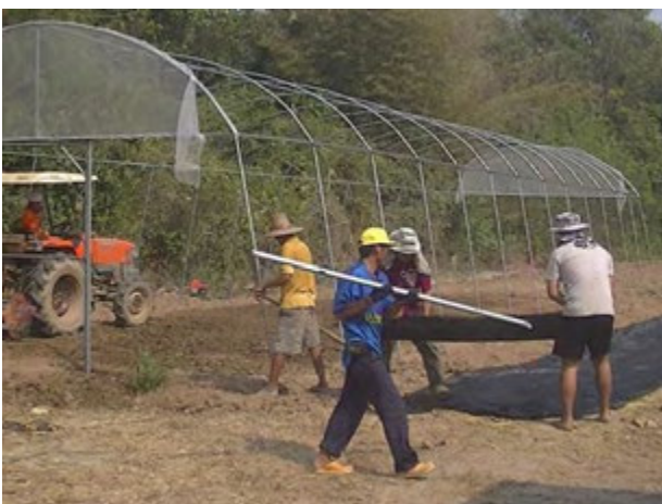
A Type-A net house, a complete set made of steel pipes and plastic sheet, was constructed. (Jan. 24, 2013)
