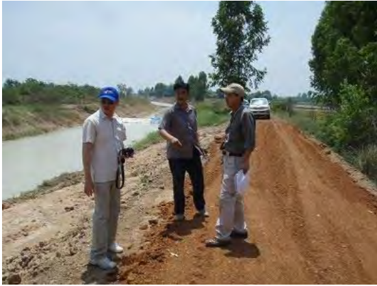
The length of 1.3 km laterite pavement with 10 cm thickness was paved completely.
