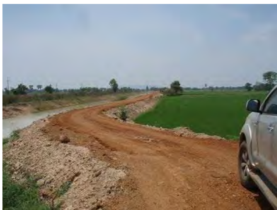
Final inspection was carried out in the presence of TAO staff and JICA Study Team on 20 th March 2013.
