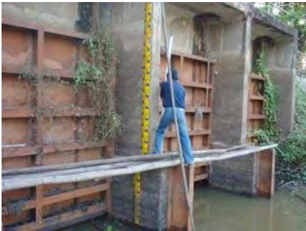
Installed staff gage
