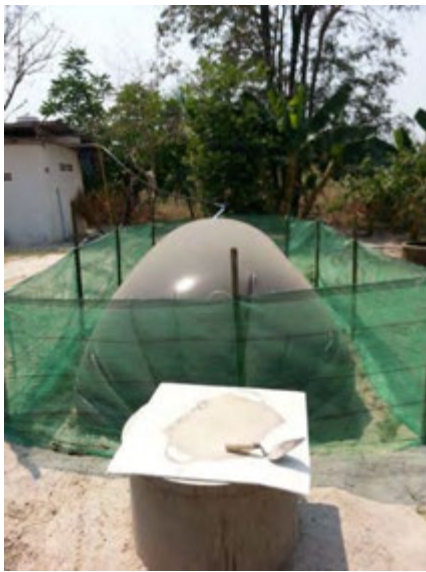
The inlet tank
