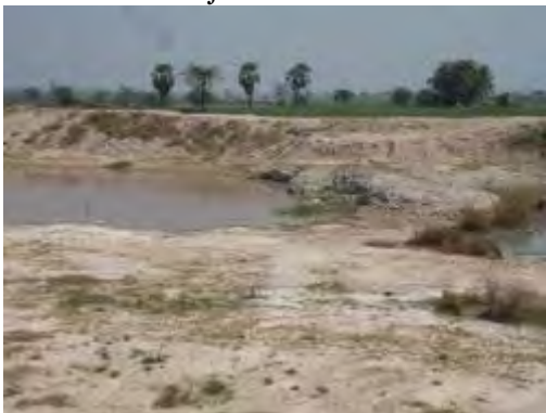
Slope of the pond is not well constructed.
