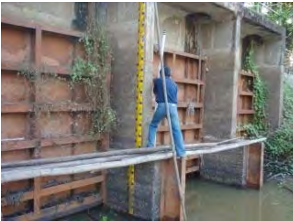
Installed staff gage
