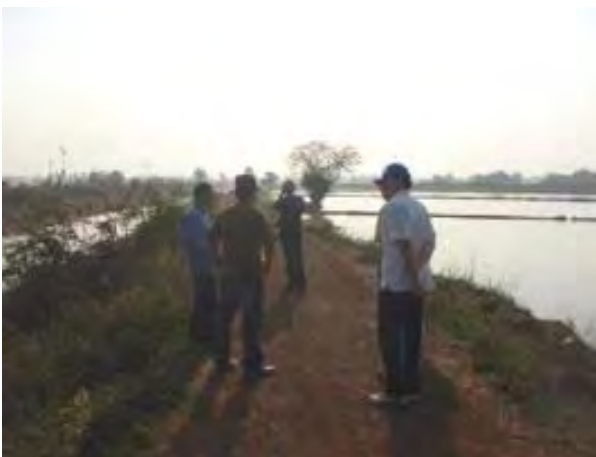
Repairing dike Left; drainage canal, right; paddy field where is damaged by overflowing from drainage canal annually., 6ht February 2013
