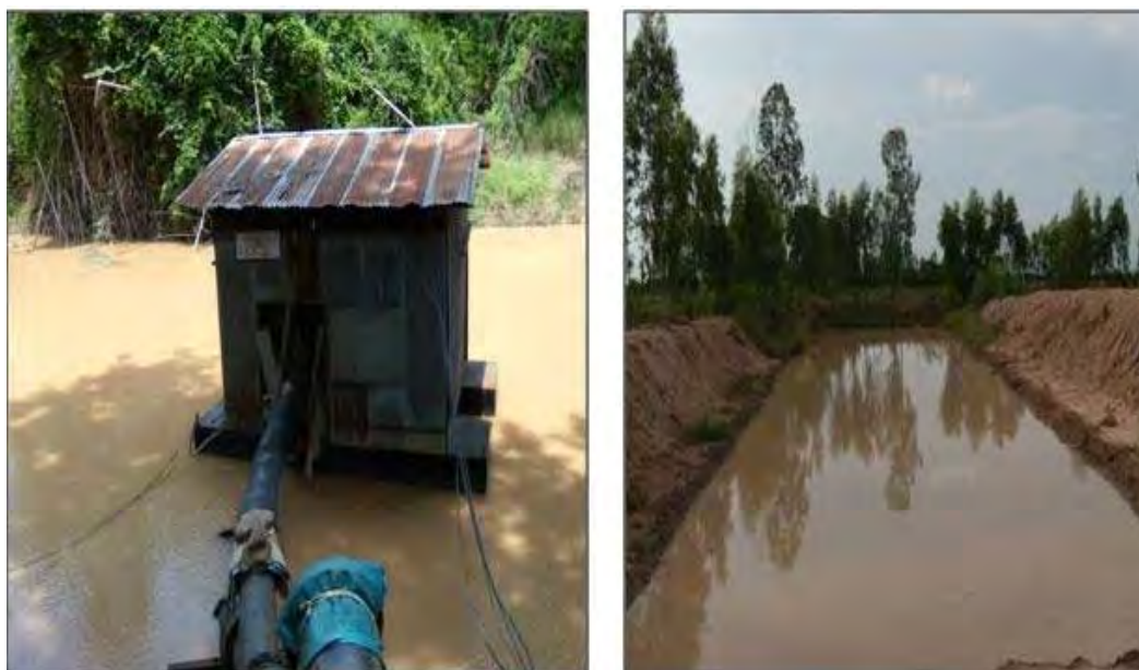
Figure 16 Electrical Pumping Station and Swamp in the Rice Field
