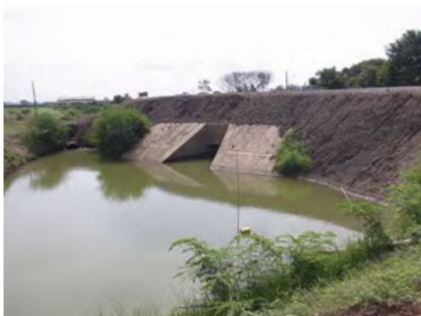
After the flood of 2011, elevation of dike was elevated No. 2 and 3 are located outside of Monkey Cheek.
