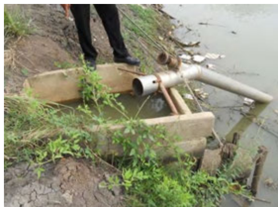
Water needs to be pumped up from the canal; the canal is used both for irrigation and drainage.
