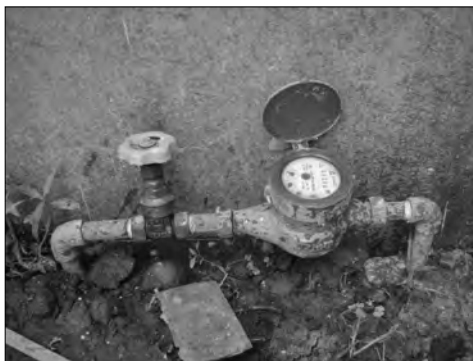
Installed water meter
