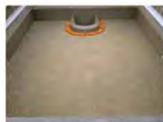
1. Before cleaning The state of lack of filtration due to mud or algae
