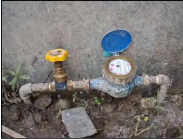
Photo-3 Installed water meter
