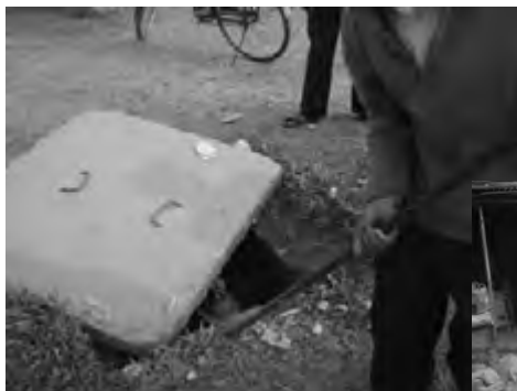
Gate valve chamber
