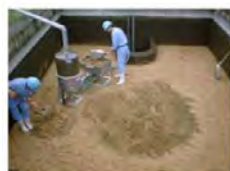
4. Cleaning with sand washer Cleaning the scrapped sand by sand washer with high pressure water
